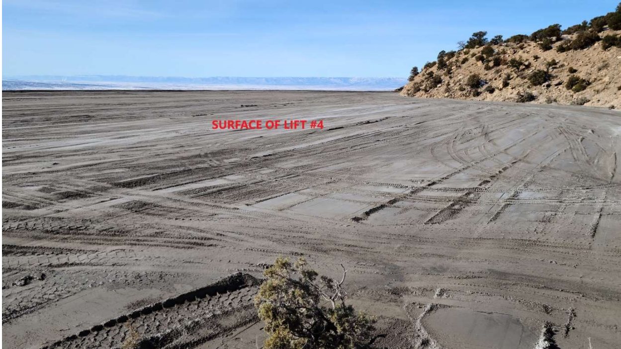
Surface of Lift #4 in process – photo looking northwesterly January 14, 2021 Compaction appears satisfactory. Dust suppression appears satisfactory
