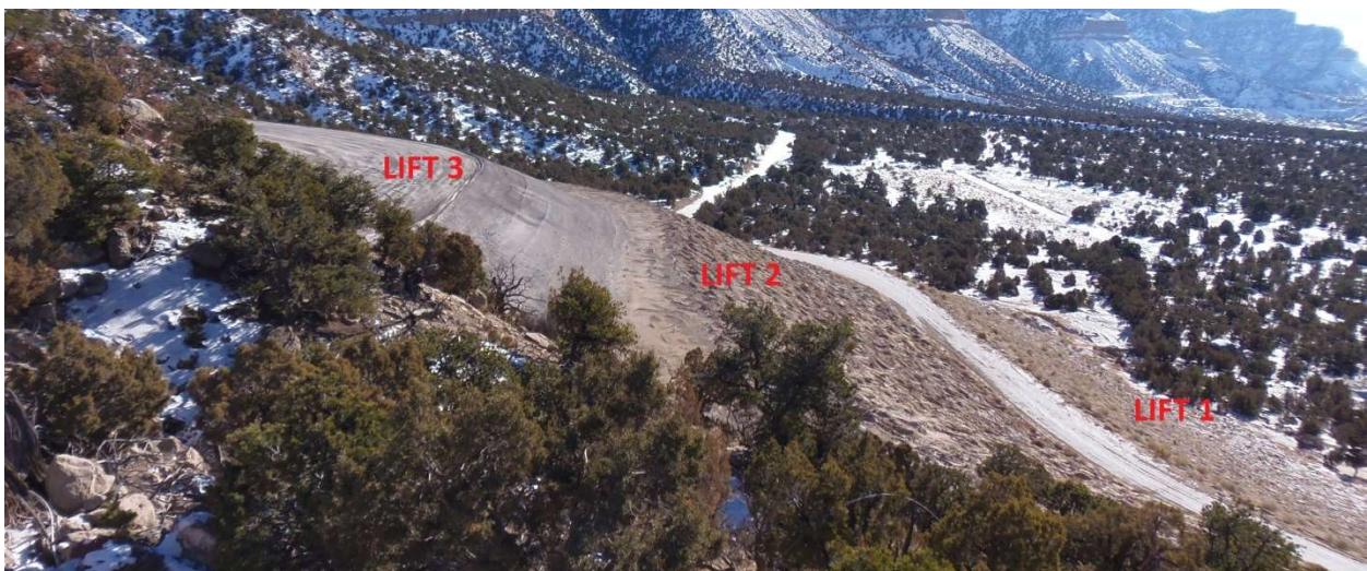
SCA#2 Ash Landfill – west face looking southerly Lift #1 and #2 covered and seeded, vegetation is growing. Lift #3 in process
